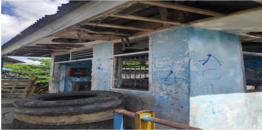
Gambar 4.8 Ruang Operator Movable Bridge
