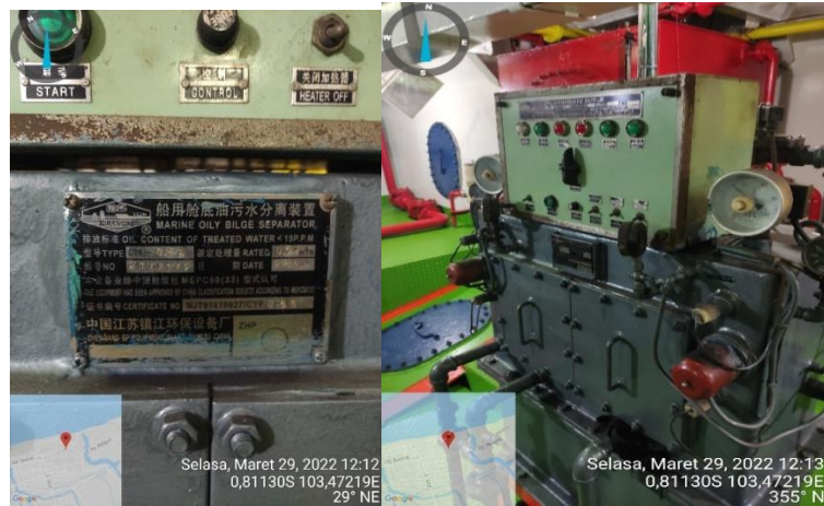
Gambar 4.51 Oily Water Separator KMP Sembilang
